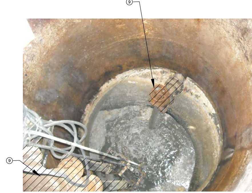
ANCHOR PUMP STATION WETWELL INLET PIPING
