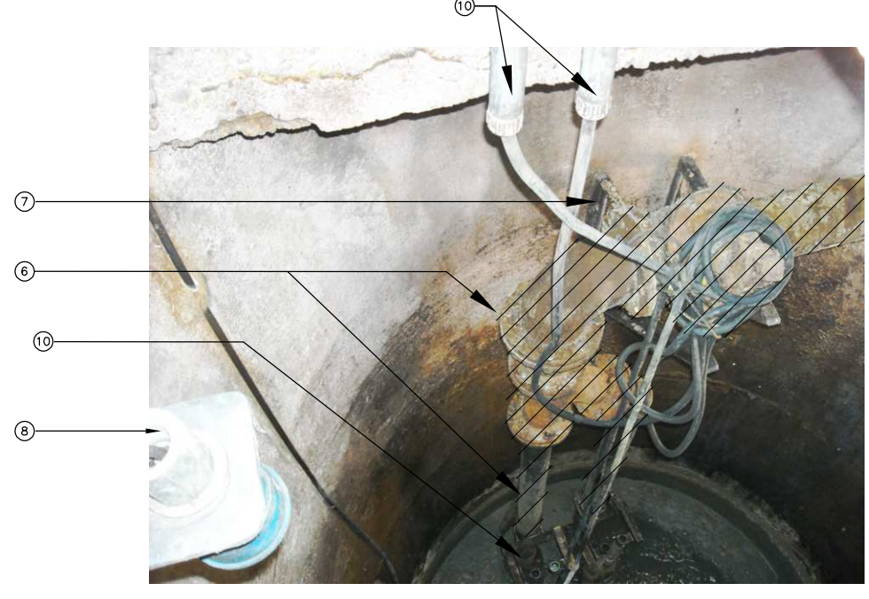
ANCHOR PUMP STATION WETWELL INTERNAL PIPING
