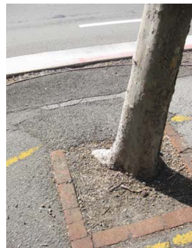
Tree roots on the existing Bridgeway sidepath are pushing up the asphalt path
