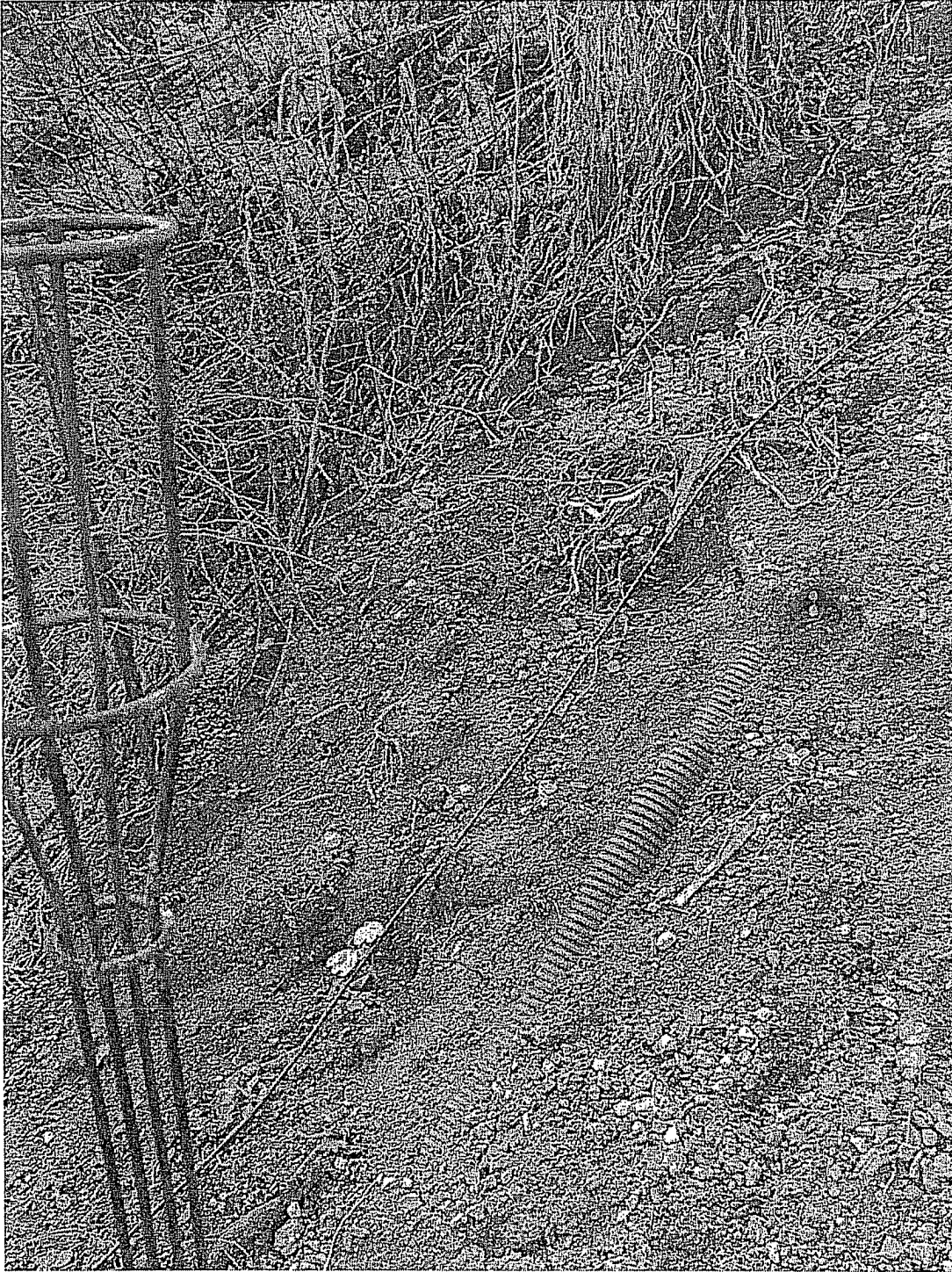
Image 3 – Encroaching Plastic Drain Pipe
