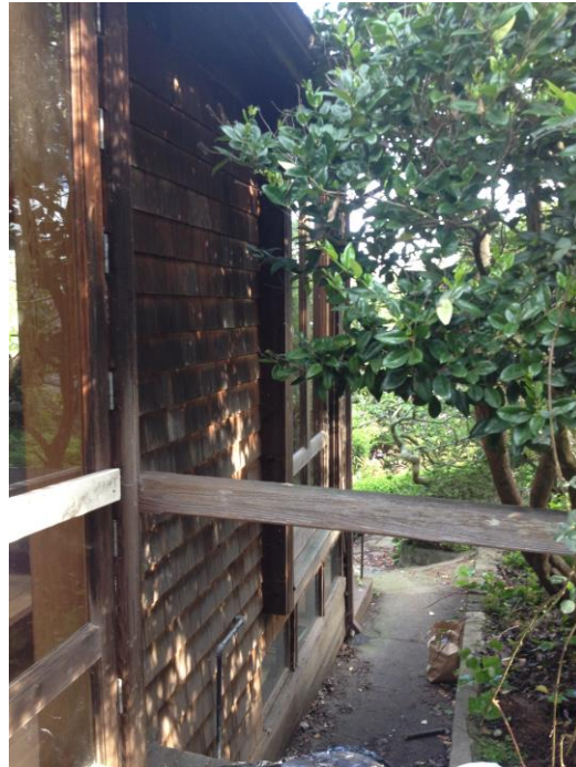
Figure 17. North portion of southeast façade, looking north from elevated wood deck. Basement level windows and first story window at center.
