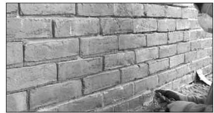
Repoint mortar joints where there is evidence of deterioration.
