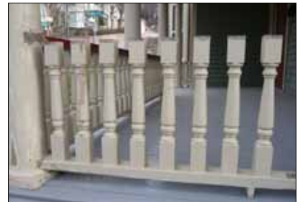
When replacing a missing feature, use the same kind of material as the original.
