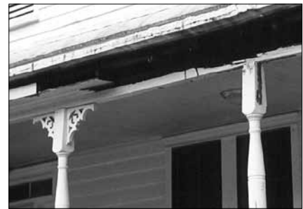
Replace missing original details in kind.
