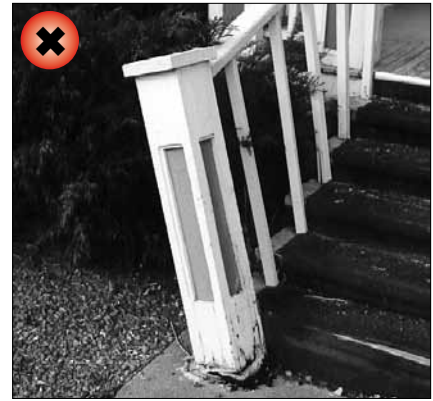
Before: A deteriorated railing should be repaired rather than replaced.
