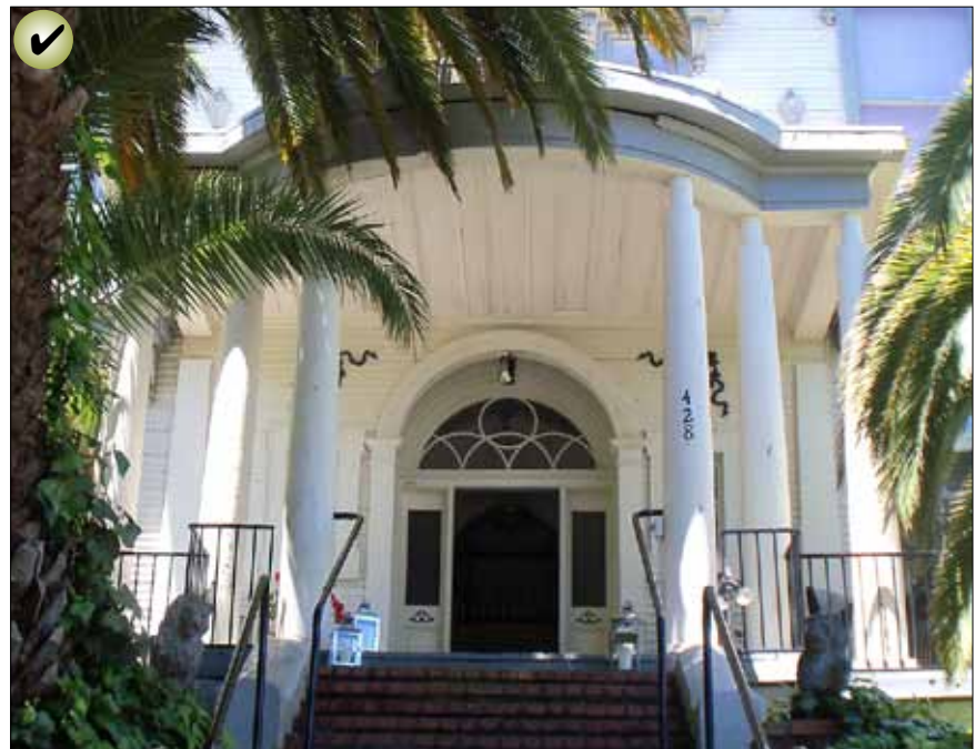
Maintain the original proportions of a significant door. This includes the transom and sidelights.
