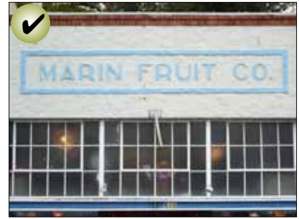
Historic signs, such as this one mounted and painted on the exterior of a building, should be preserved.
