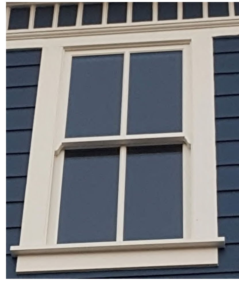
ALL (N) WINDOWS & FRENCH DOORS TO MATCH (E) WINDOWS IN MATERIALS, FINISHES, COLORS, OPERATION (DOUBLE-HUNG) MULLIONS AND FRAME STYLE. SEE ELEVATIONS ON A3.3 FOR HEAD TRIM, TYP.
