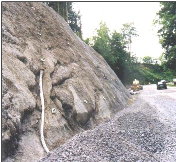
Example: Drainage hose to drain arising hillside water
