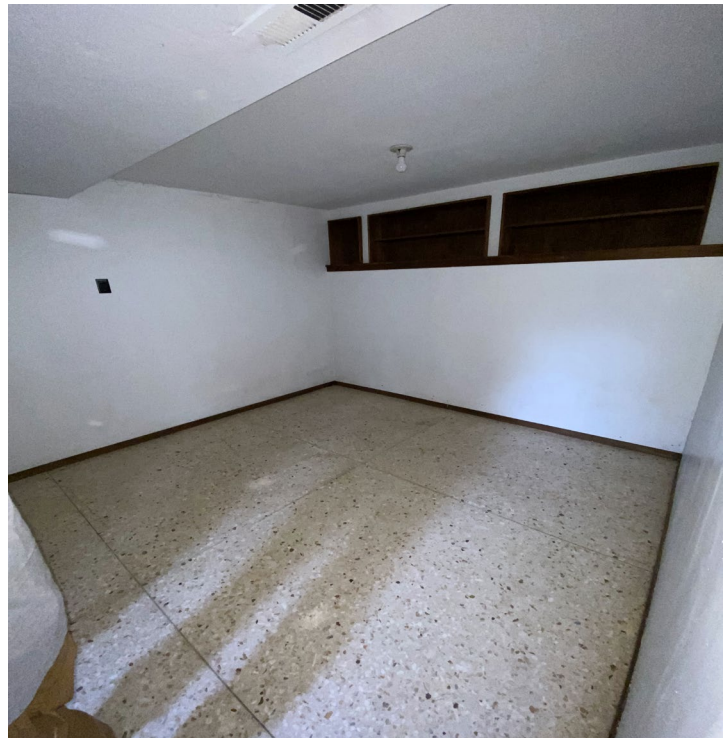
Downstairs unit. Location of relocated bathroom to be against wall that current has shelving. Required plumbing to be included in scope.
