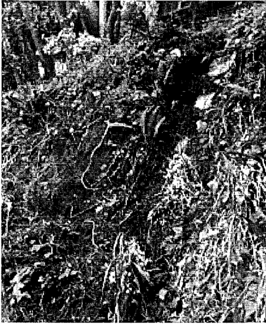
Erosion above 199 Santa Rosa Ave
