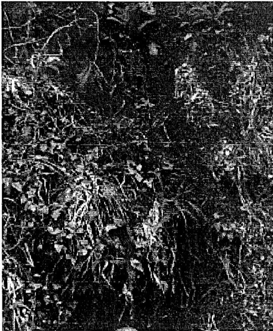
Erosion above 199 Santa Rosa Ave
