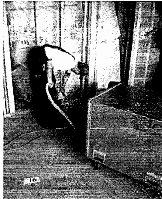
Hepa Vacuuming and wiping, dehumidifiers, and air purification for final stage of mold remediation
