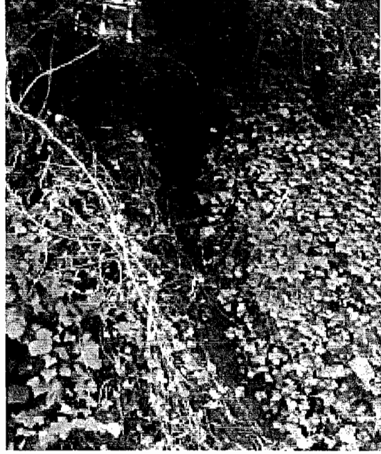
Erosion above 195 and 199 Santa Rosa Ave
