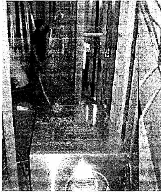
Hepa Vacuuming and wiping, dehumidifiers, and air purification for final stage of mold remediation
