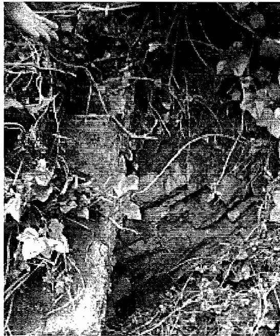
Rock/Limestone surrounding Pole that would have to be bored through to trench up the hill
