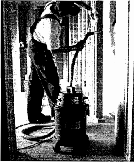
Hepa Vacuuming and wiping, dehumidifiers, and air purification for final stage of mold remediation
