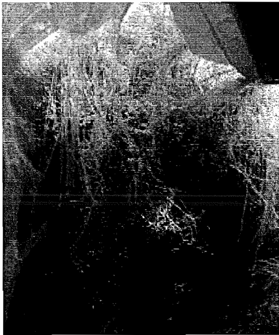
tarping torn from blowing in the wind and contractor abandoning site
