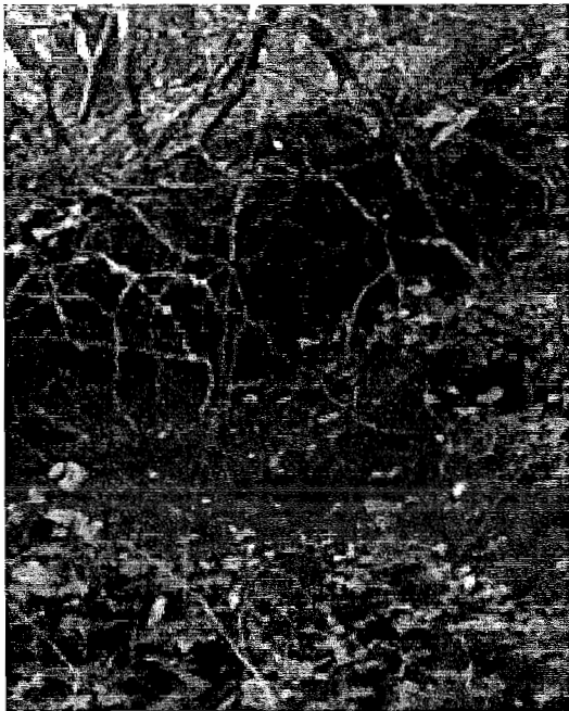
Erosion below 203, 207, 211 Santa Rosa Ave
