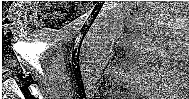
Understand the soils and deal with the settlement issues.
