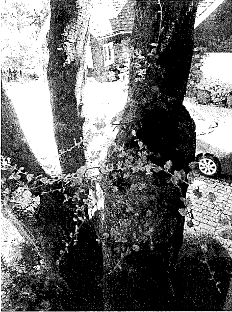
Picture 2. Large pocket of decay on stem that hangs over the garage.
